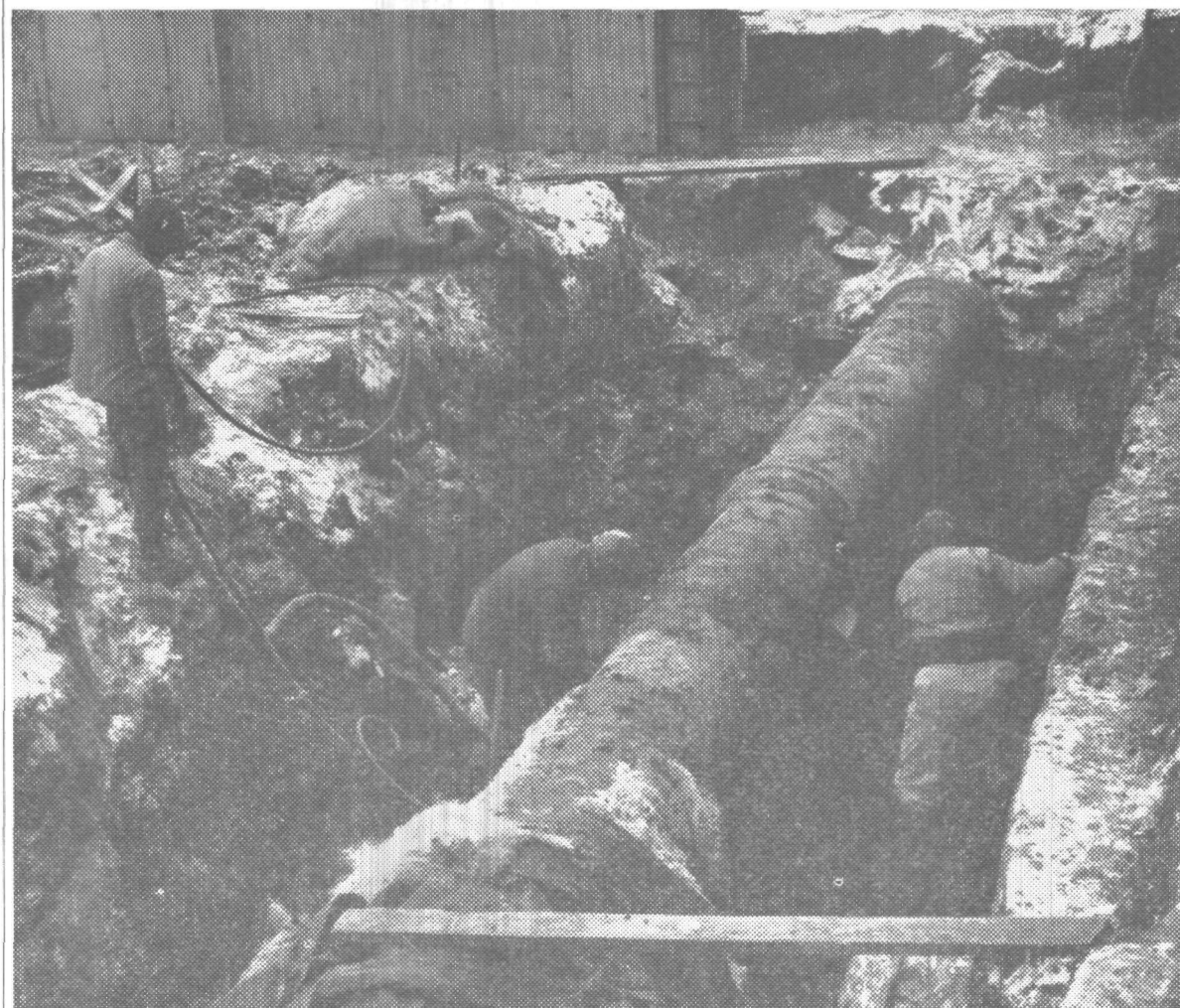
DIGGING A TUNNEL —Workmen dig around the 24-inch water main, which carries all of the plant's water supply, in preparation for construction work on a new building to go in just east of 34 Building-Warehouse. The new building will
