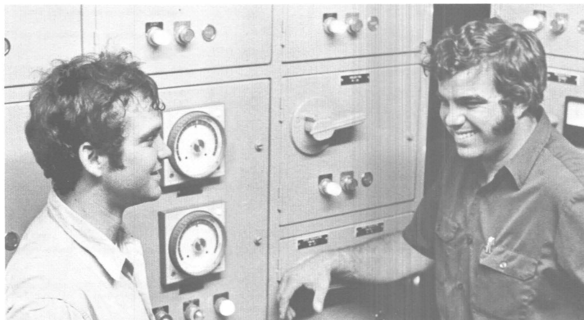
Billy Hadaway, left, operator, and Tom Barker, leadman, discuss operations in the control room at Lockport.
