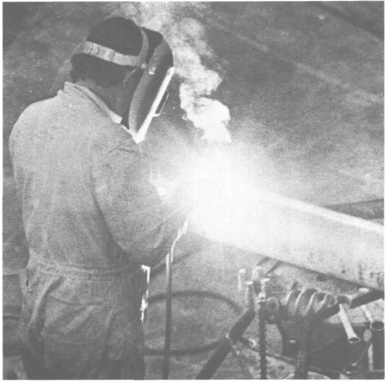
The Morrisville expansion progresses and sights such as this are common throughout the plant. When completed the expansion will increase Morrisville capacity for production of IsoSweet by 50 percent.
